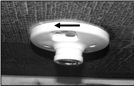
Figure 16. Ceiling mounted Type A CFL, position C1. Only the cap remains in the fixture.
